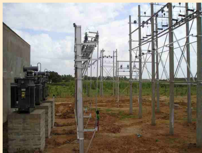
A view of the electrical distribution system being set up, Kabbigere (Koratagere)
