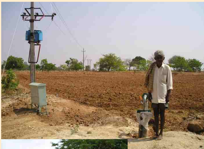
▲ Borewell with OYT Transformer, Kabbigere (Koratagere)
